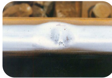
Local track defects
