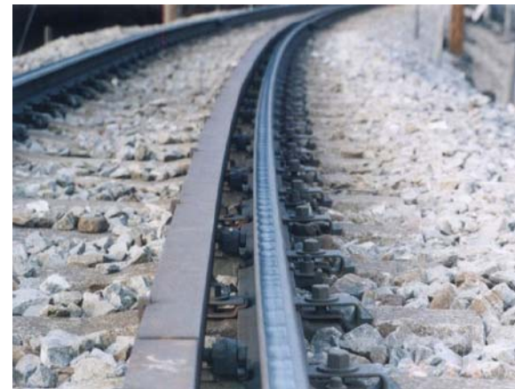
Corrugation (low rail)
