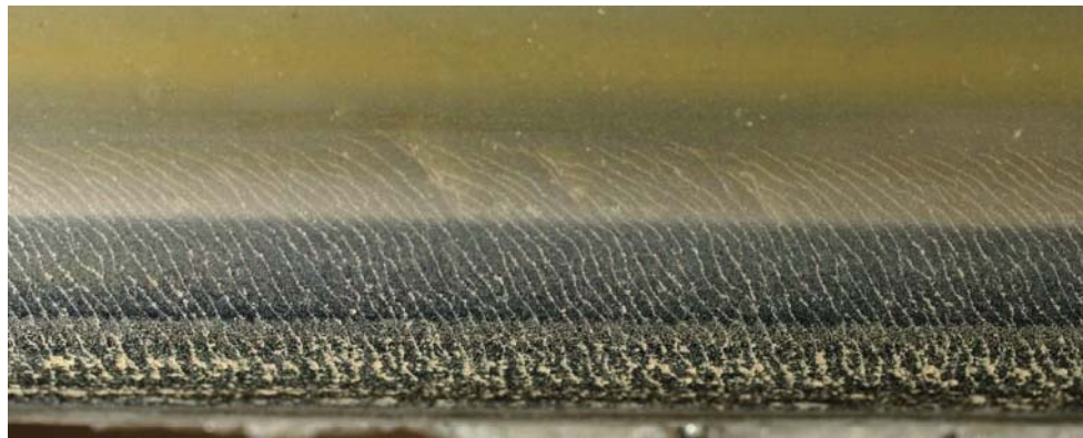
Head check (curve rail)
