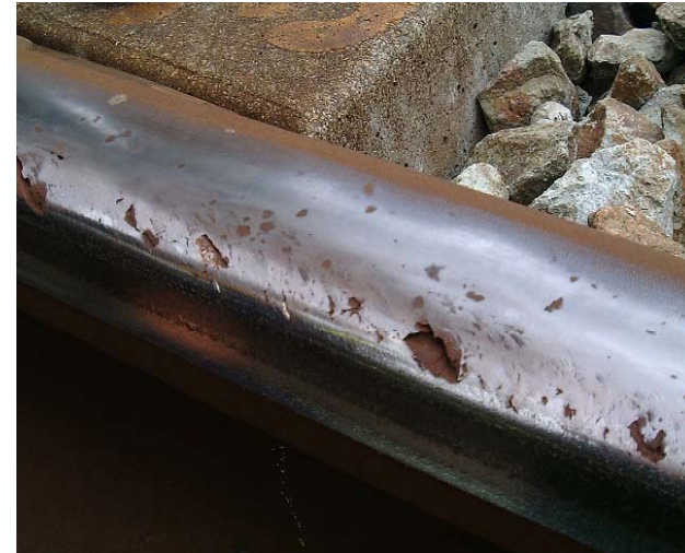
Head check & Flaking (curve rail)
