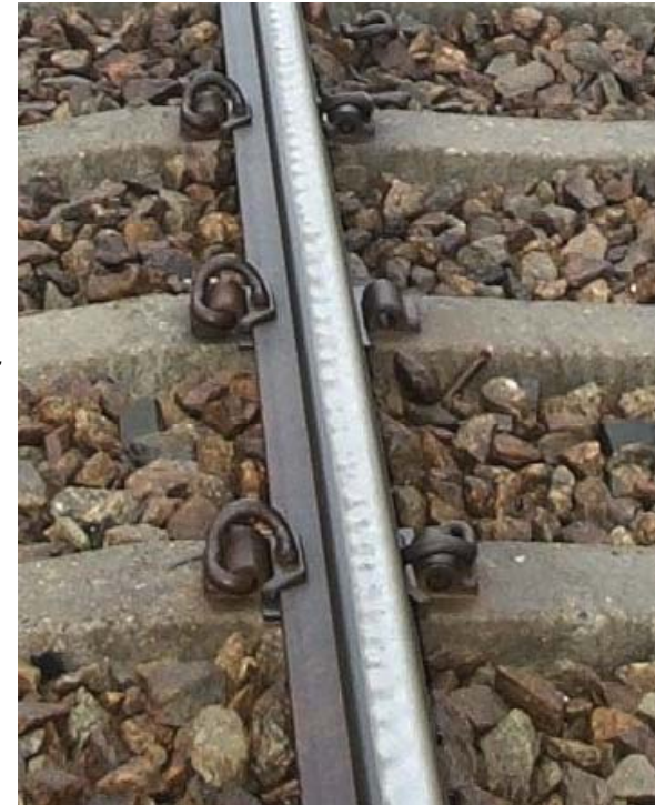
Rail corrugation Photo Lennart Lundfeldt, Banverket
