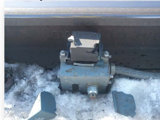
Failed sensor belonging to the wheel profile monitoring system (photo by Dan Larsson).
