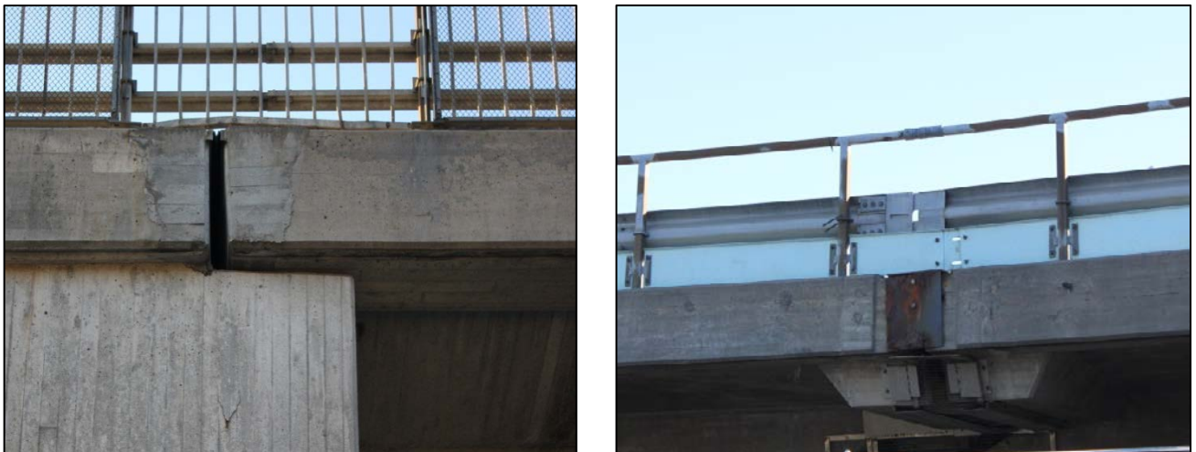
Figure 1.9: Faulty expansion joints causing excessive movements at the edge beam can also create cracks and damage to the edge beam
