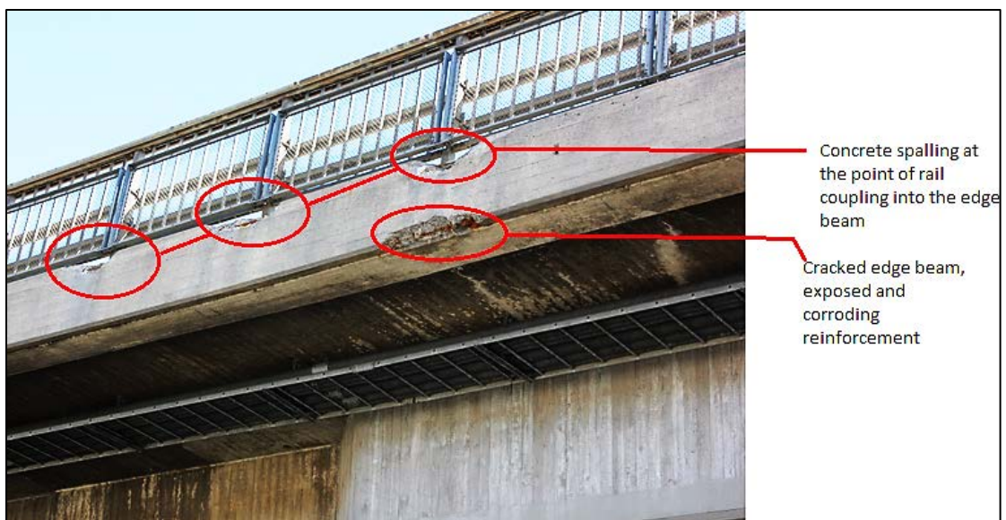
Figure 1.7: Cracks, corrosion and degradation in BEBS
