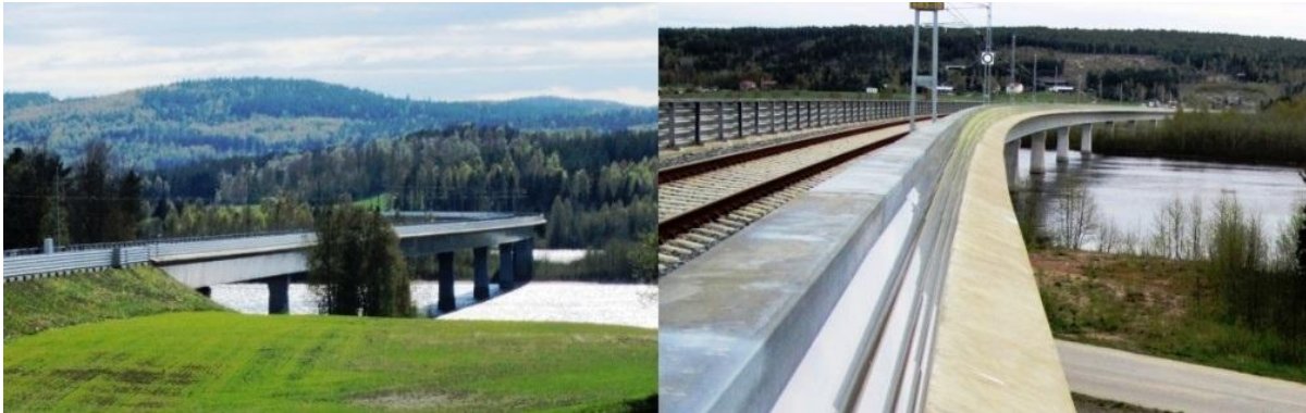
Figure 1.2 Photo of the Ångermanälven Bridge from north side (left) and south side (right).
