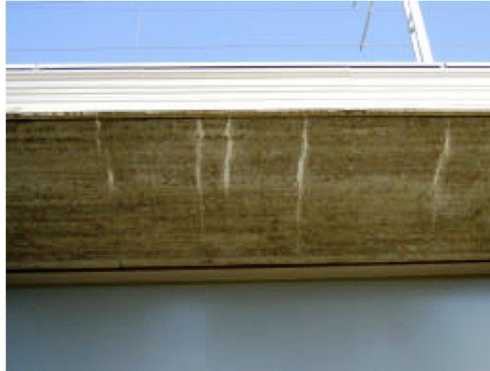
Figure 2.19 Cracks at support 16, left side (Carlsson, 2008).
